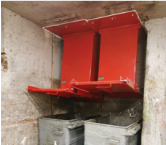
A 240 min fire-rated chute discharge pipe/ chute extension is required when no fitting directly to the FCP directly to the ceiling slab. (Illustrated)
